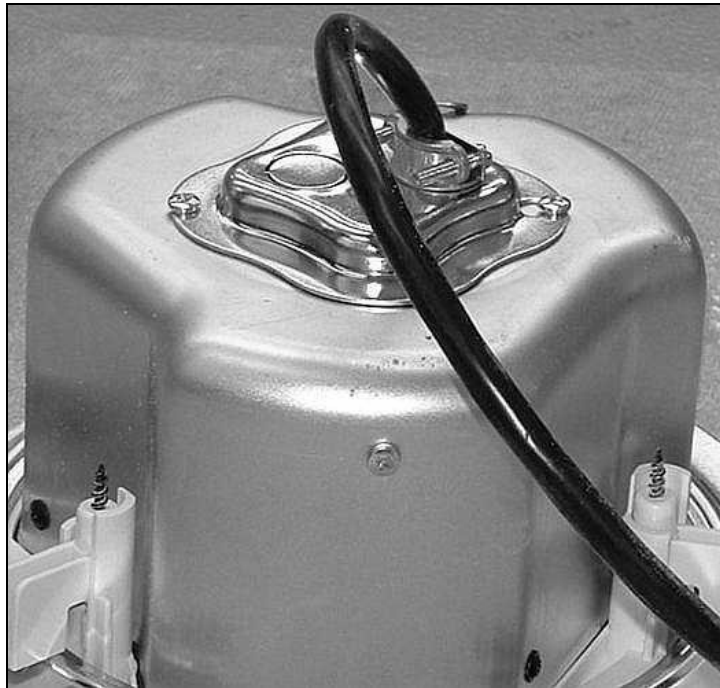
Ceiling loudspeaker rear can – fireproof steel cover fitted
