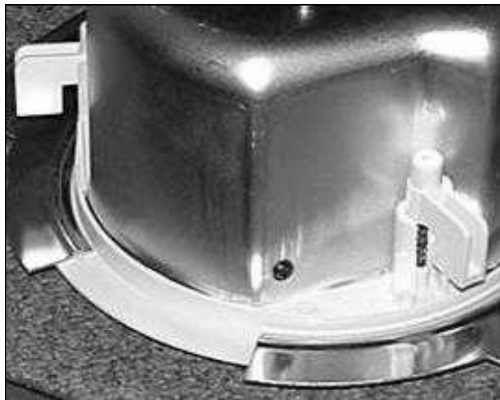
Loudspeaker in place.
