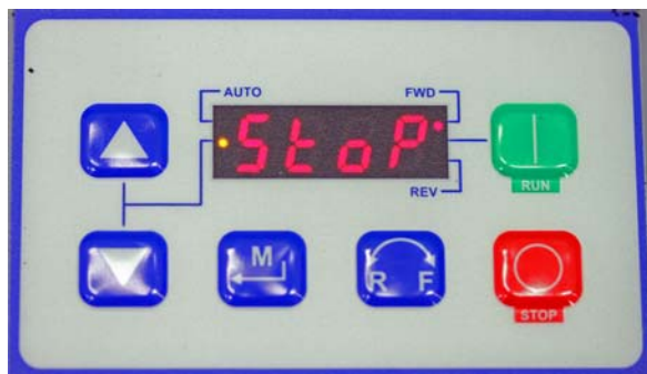
Figure 15 VFD Control Panel
